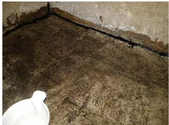
#6 Crawl space - larger cracks are sealed with suitable sealant.
