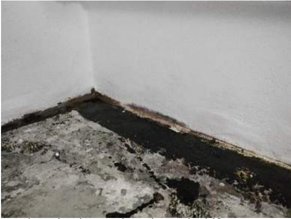
#1 Floor is cleaned and sanded if necessary before edges are sealed with a brush.
