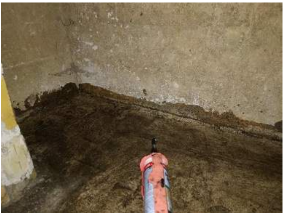
#5 Crawl space - larger cracks are sealed with suitable sealant.
