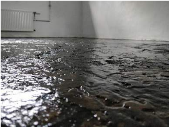
#3 After approx. 24 hours, the membrane is cured and the floor can be further treated.
