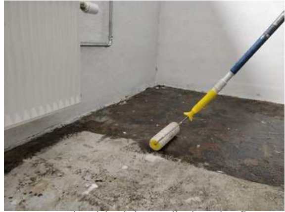
#2 SPS Radon block is applied to the floor surfaces with a roller.
